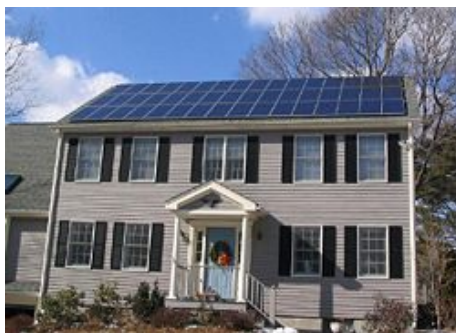
Example of roof-mounted photovoltaic modules.
